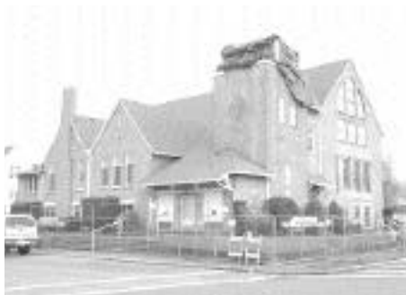
Tarps cover the damaged bell tower at United Methodist Church.
