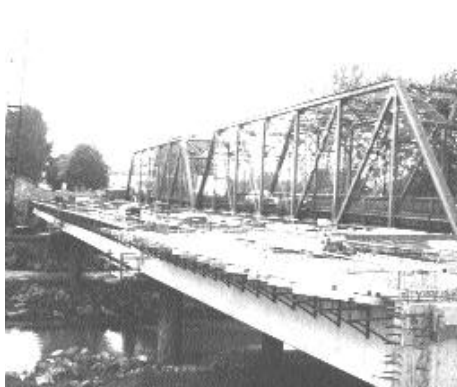
The existing two-lane steel structure is being replaced by a concrete span.
