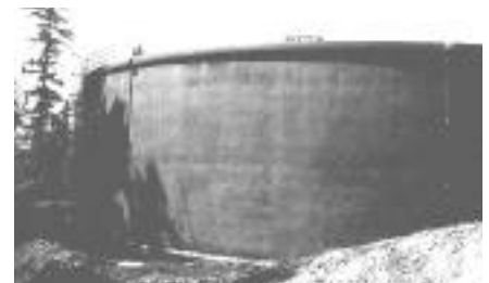
The new two-million gallon reservoir is on a bluff in northeast Sumner.
